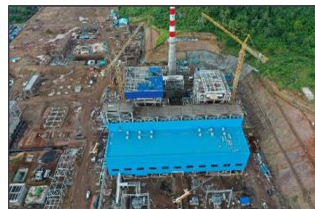
MCL Main Power House
