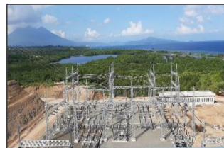
MCL Substation 150 KV
