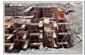
GLP CW Pump House
